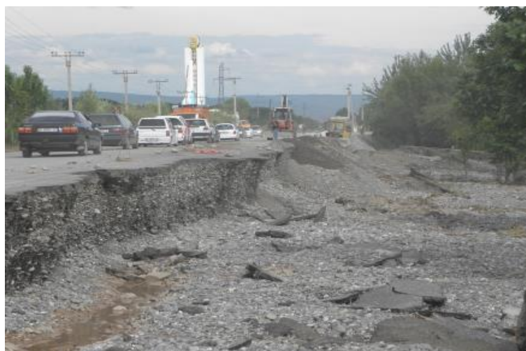
Figure 1. Consequences of floods in the Kara-Unkyur-Sai River, June 5, 2010.
